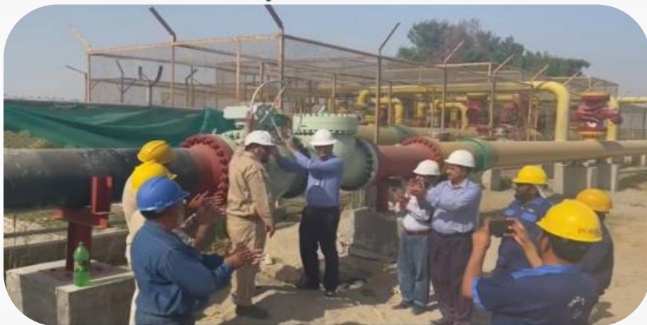
20" x 25 km Cross Country Pipeline SNGPL Custody Transfer Point
