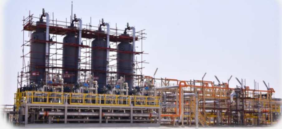
Tipu Gas Processing Plant
